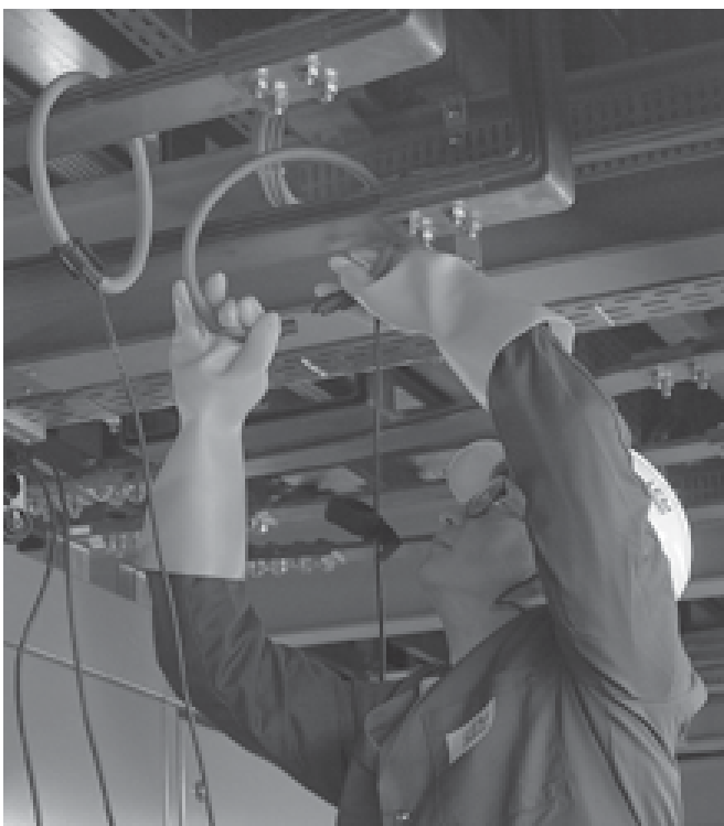
Fig. 40 Typical LEM-flex use, surrounding conductor(s) and latched.
