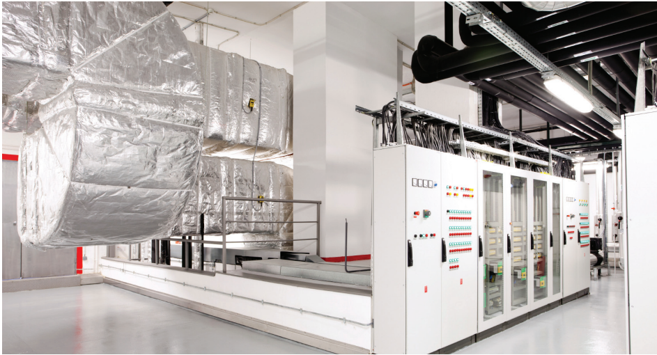
Technical floor of a smart building HVAC system.
