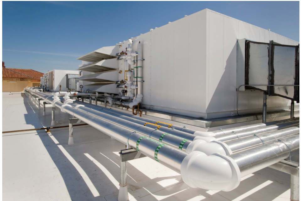
Rooftop unit part of HVAC system for large commercial building.
