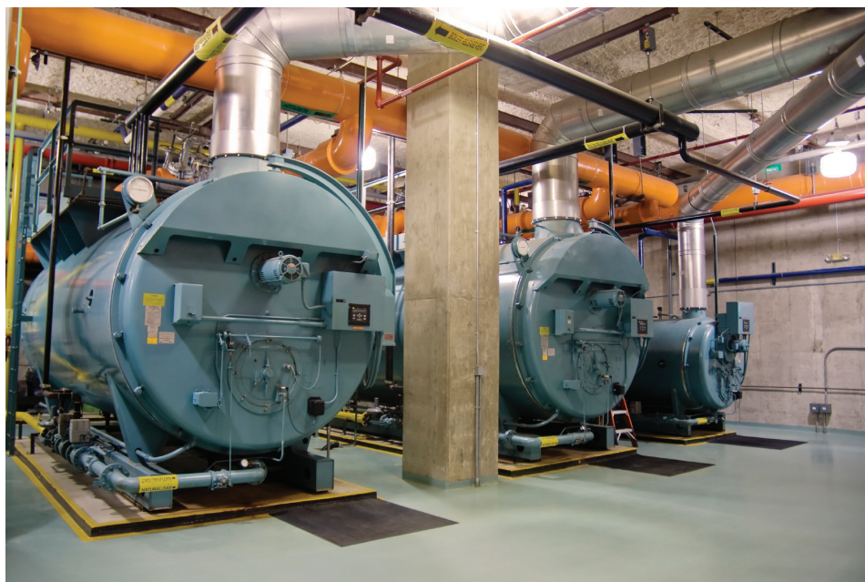
Boiler room in a commercial facility.
