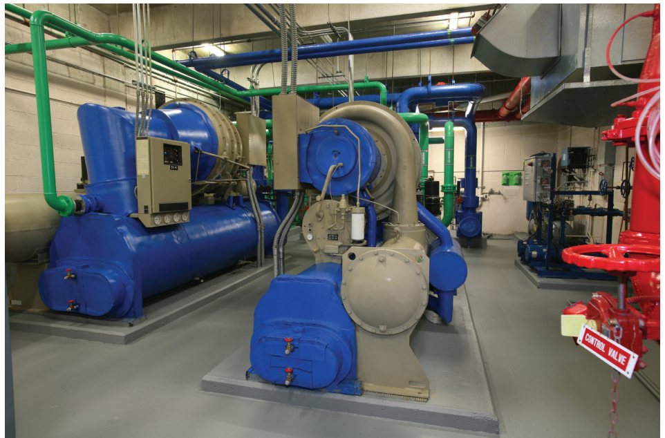
Chiller room for a building cold water system.
