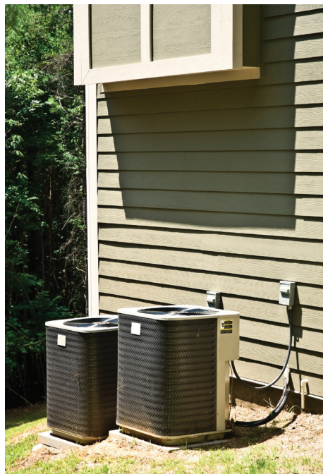
Home air conditioner.
