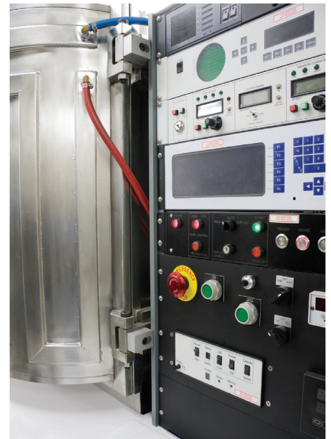
Control panel with a variety of input and output types.
